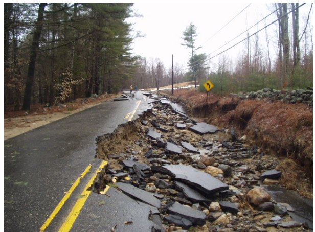
Route 109 in Acton, ME after April 2007 flooding. Photo courtesy of Maine DOT.
